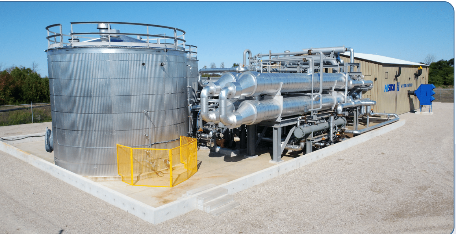
SOURCE: Hydrostor ( https://hydrostor.ca/projects/the-goderich-a-caes-facility )
